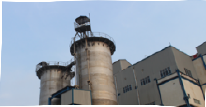
Storage Chip / Silo
