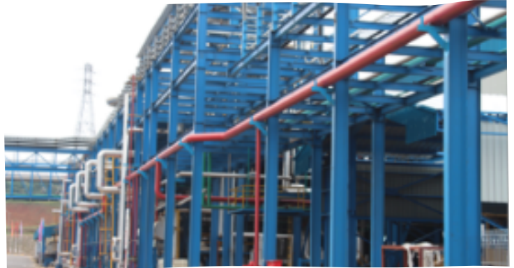
Utility Pipe Rack
