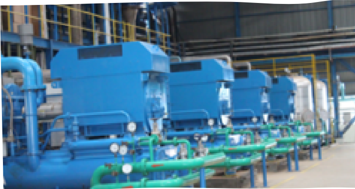
Compressor Room & Piping
