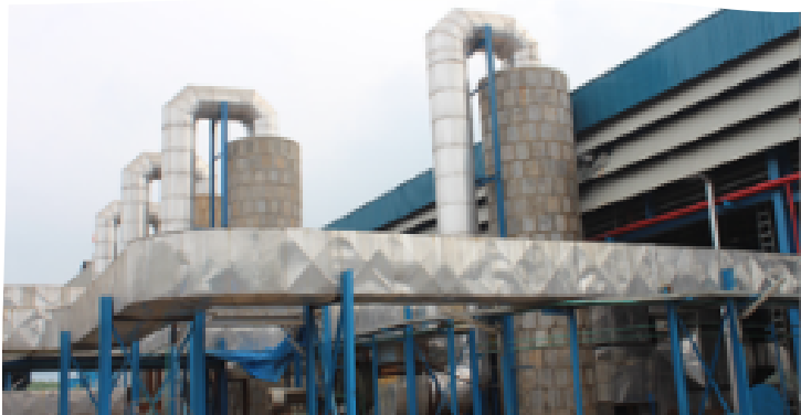
Wet Scrubber & Ducting
